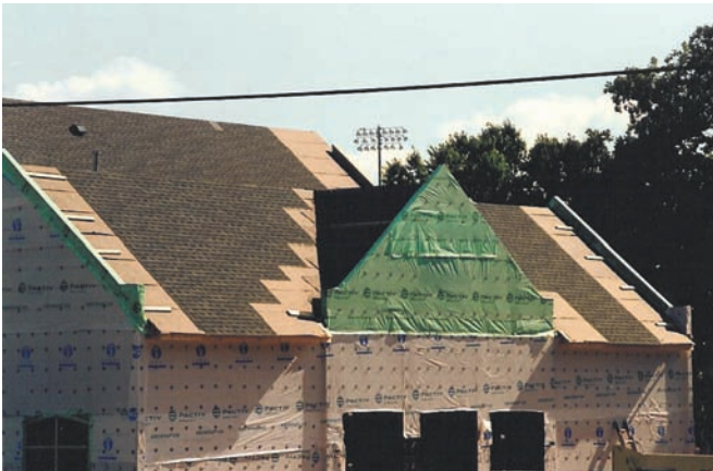
Figure 3 and 4: The photo at left shows racked shingles. The one below shows the correct way to lay shingles.
